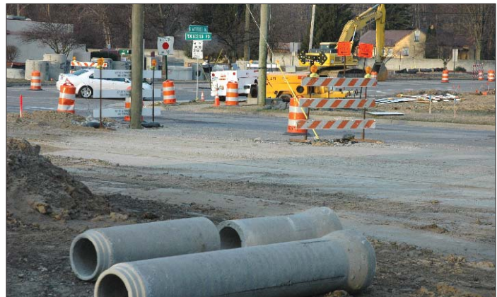
The road construction and widening project on Rochester and Wattles Roads started in February and will continue through the summer of 2010. More details about this and other road projects are on pages 10-11.
